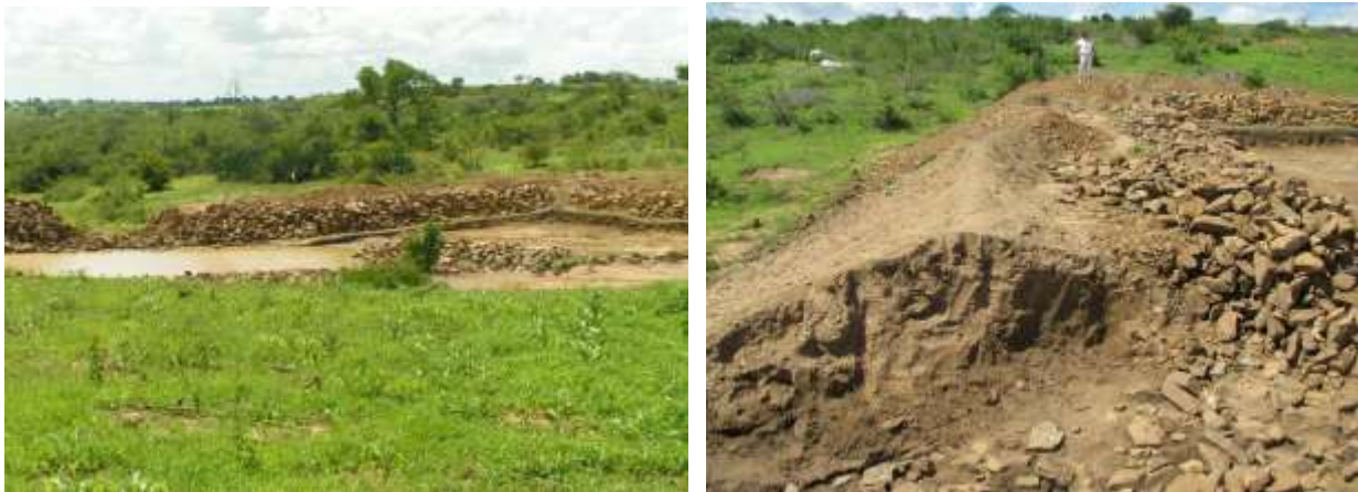
Photo 10 Pond dug for water retention after levy failed.
