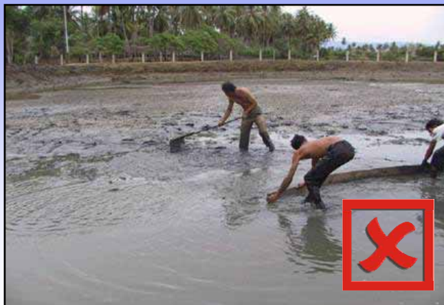
Improper removal of black soil
