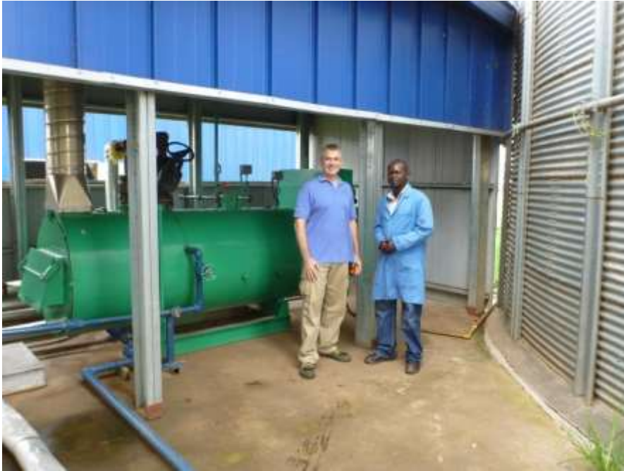
Steam Boiler for Dominion Farms (Lukas, Wilfred)
