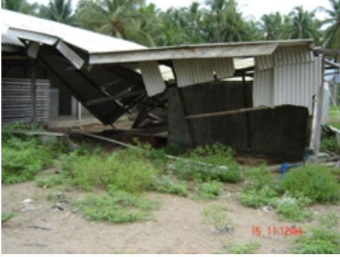
Damaged hatchery before rehabilitation
